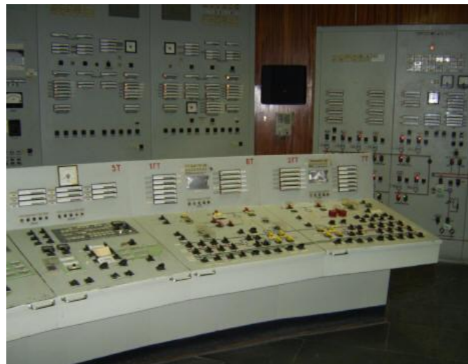
Figure 5-7: Small portion of Chernobyl nuclear power plant control room (from http://www.upandatom.net/Chernobyl.htm )
