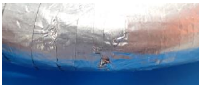
Figure 7-15: Example of not acceptable foil shielding
