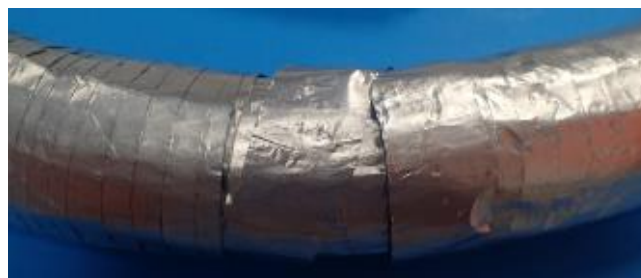
Figure 7-14: Example of not acceptable, loose foil shielding
