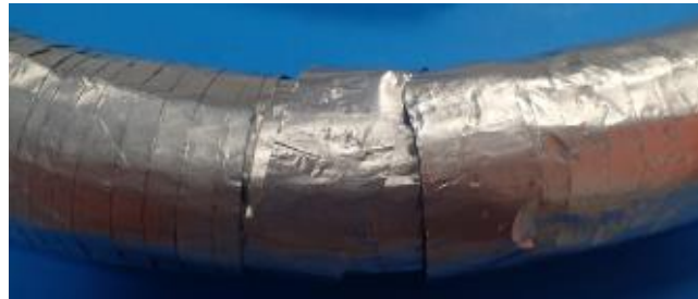
Figure 7-14: Example of not acceptable, loose foil shielding
